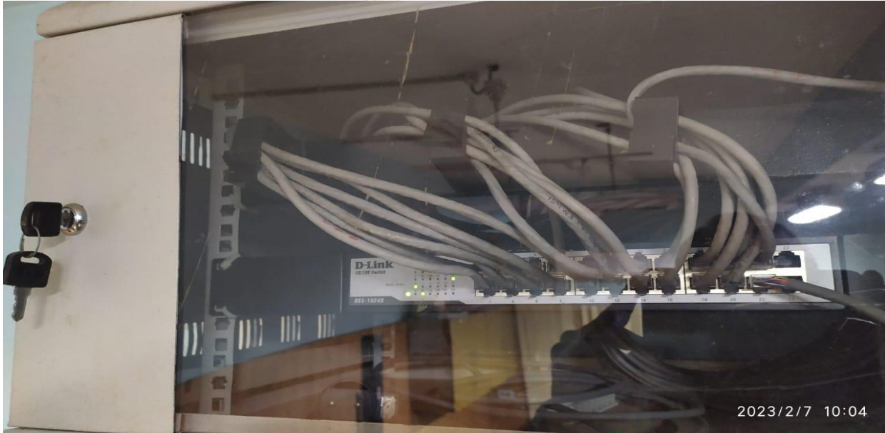
ETHERNET SWITCH IN CABINET
