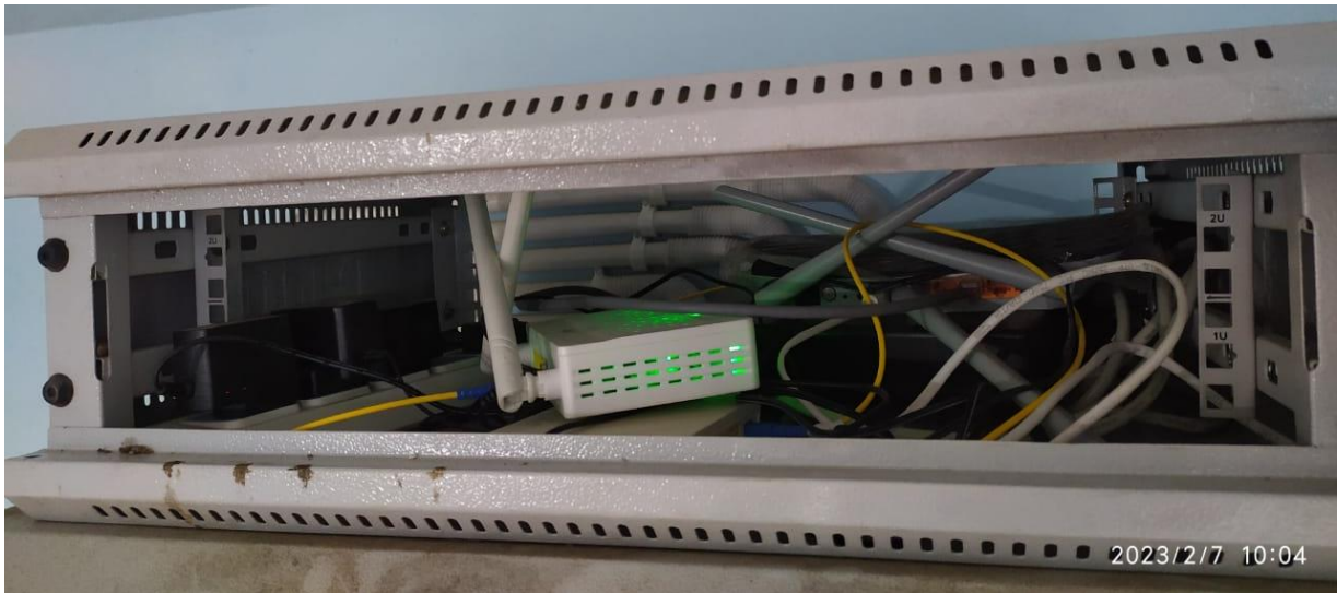
ROUTER IN CABINET
